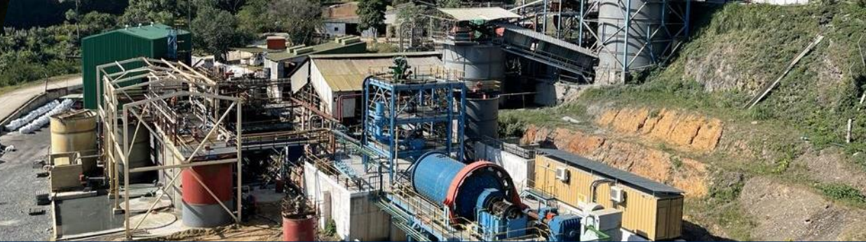
Galaxy plant today - 50,000 tonnes per month with new mill, concentrate tanks and filter press for $4m investment
