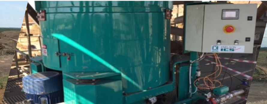
Upgraded plant to process Sulphur ore by commissioning float plant, Knelson and oxygen plant
